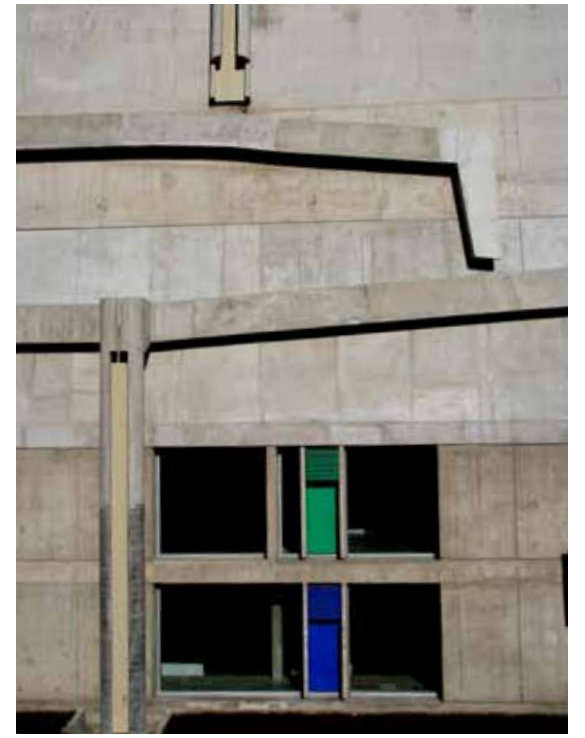
The water runs in the peripheral gutter and is led to a canal surrounding the "base" by means of a vertical shaft.
